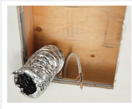
Existing 3" Duct and wiring
